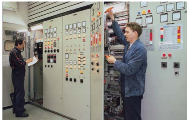
Control room for the Südtangente pumping station
