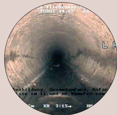
Damaged sewer before the renovation
