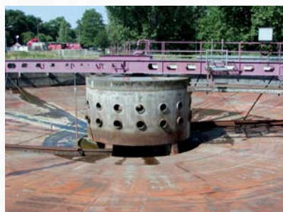
Intermediate sedimentation tank
