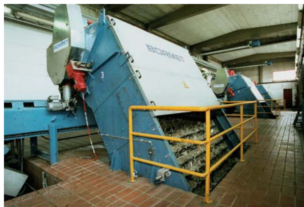
Automatic screening system, 1993
