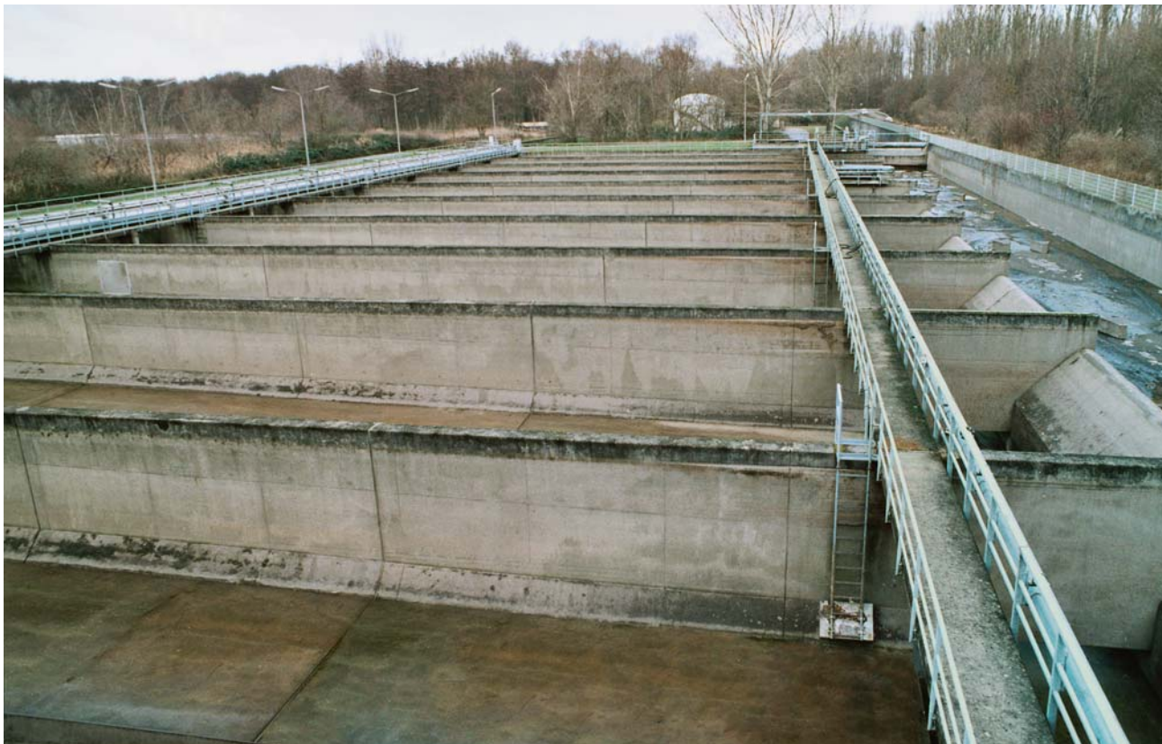
Rain overflow basins in the wastewater treatment plant with an intake capacity of 18 000 cubic metres.
