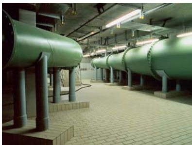
Sludge pumping station
