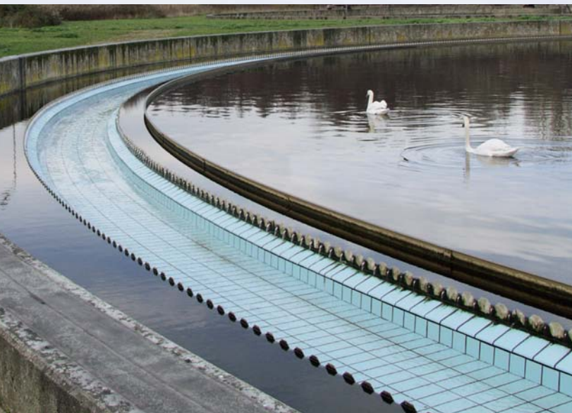
Outflow of secondary sedimentation tank
