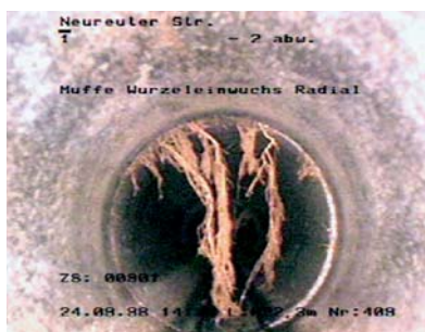
Root formation in a sewer
