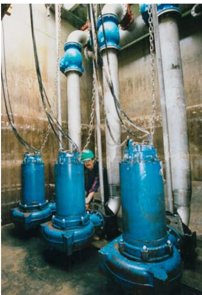
Pumping shaft with submersible pumps
